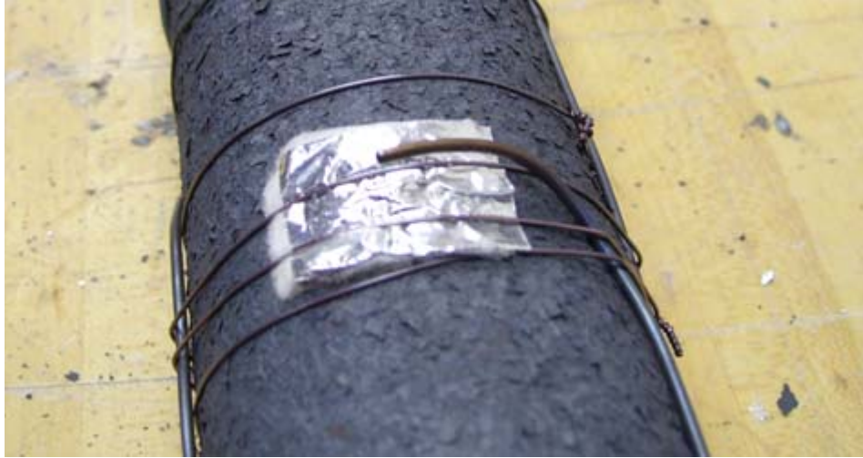
Figure 5. Absorber thermocouple with required radiant shielding on copper pipe
