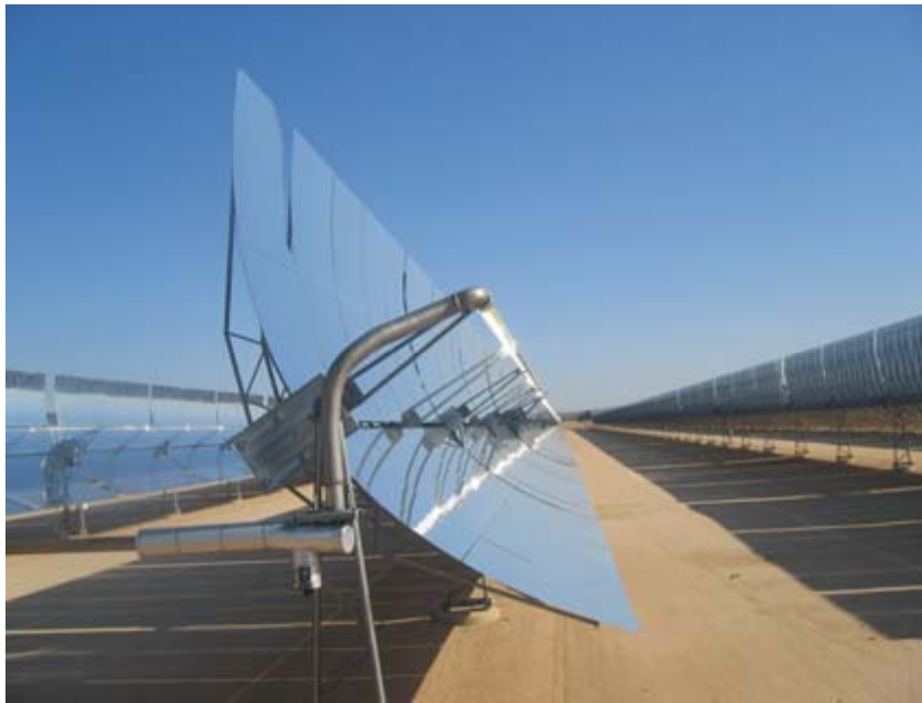
Figure 1. Mirrored trough collectors and receivers at a SEGS plant
