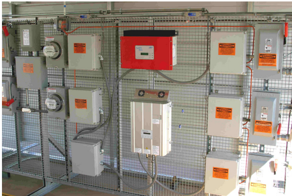
Fig. 2. PVSOL: Fully instrumented inverters in continuous system performance test
