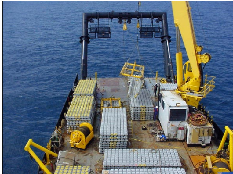
Ocean Intervention deck layout for installation of concrete mattresses over pipeline & umbilical crossings.
