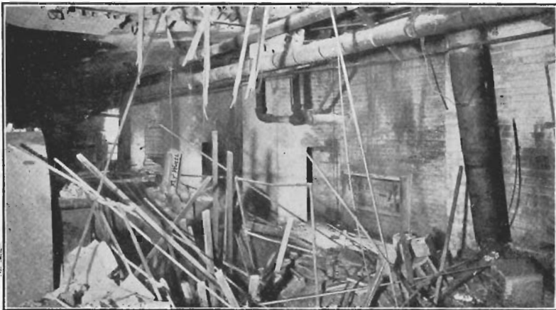
FLY-WHEEL EXPLOSION, BRADLEY ELECTRIC LIGHT, HEAT AND POWER CO., CLEVELAND, O. BELT BROKE AND WRECKED GOVERNOR; ENGINE RACED. LOSS $4,000. WHEEL INSURED.
