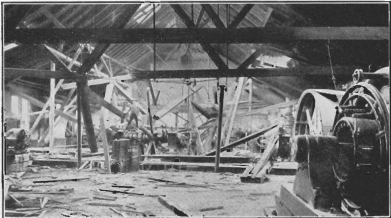
FLY-WHEEL EXPLOSION, MANSFIELD RAILWAY LIGHT AND POWER CO., MANSFIELD, O. BELT BROKE AND WRECKED GOVERNOR AND SPEED LIMIT, AFTER WHICH ENGINE RACED AND EXPLODED WHEEL BY CENTRIFUGAL FORCE. ONE PERSON INJURED; PROPERTY LOSS $9,000; WHEEL INSURED.
