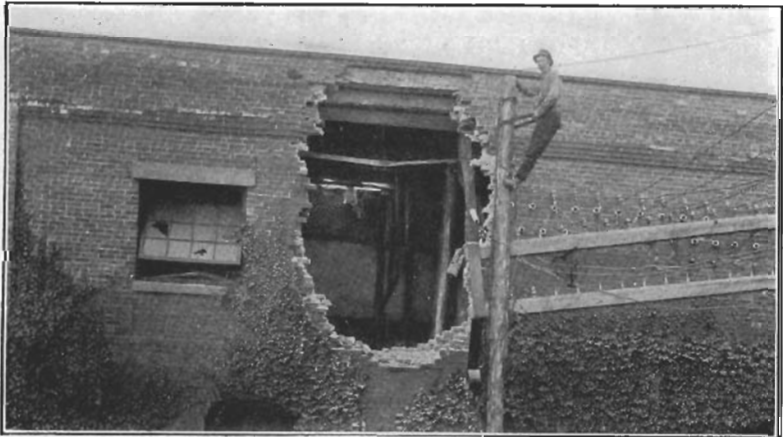
FLY-WHEEL EXPLOSION, SAYRE ELECTRIC CO., SAYRE, PA. ENGINE AND DYNAMO WRECKED. BUILDING DAMAGED. LOSS $8,210. VIEW SHOWS WHERE LARGE SEGMENT WAS HURLED THROUGH WALL. WHEEL INSURED.
