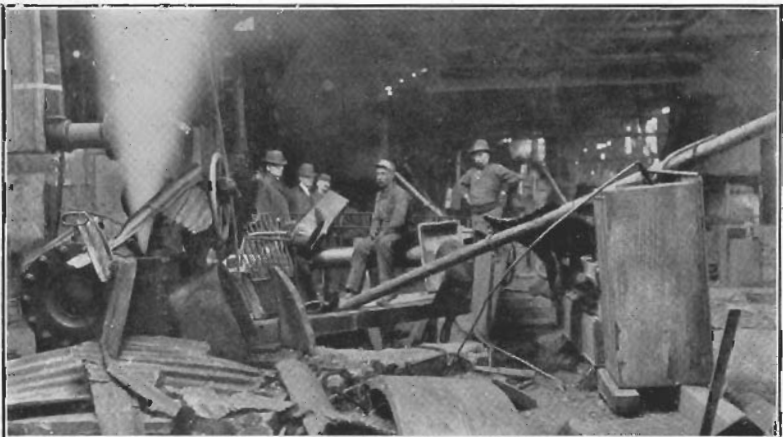
FLY-WHEEL EXPLOSION, NATIONAL ROLLING MILL CO., VINCENNES, IND. CYCLONE BLEW DOWN STACK WHICH FELL ON GOVERNOR, CAUSING ENGINE TO RACE AND BURST FLY-WHEEL BY CENTRIFUGAL FORCE. LOSS $1,900.
