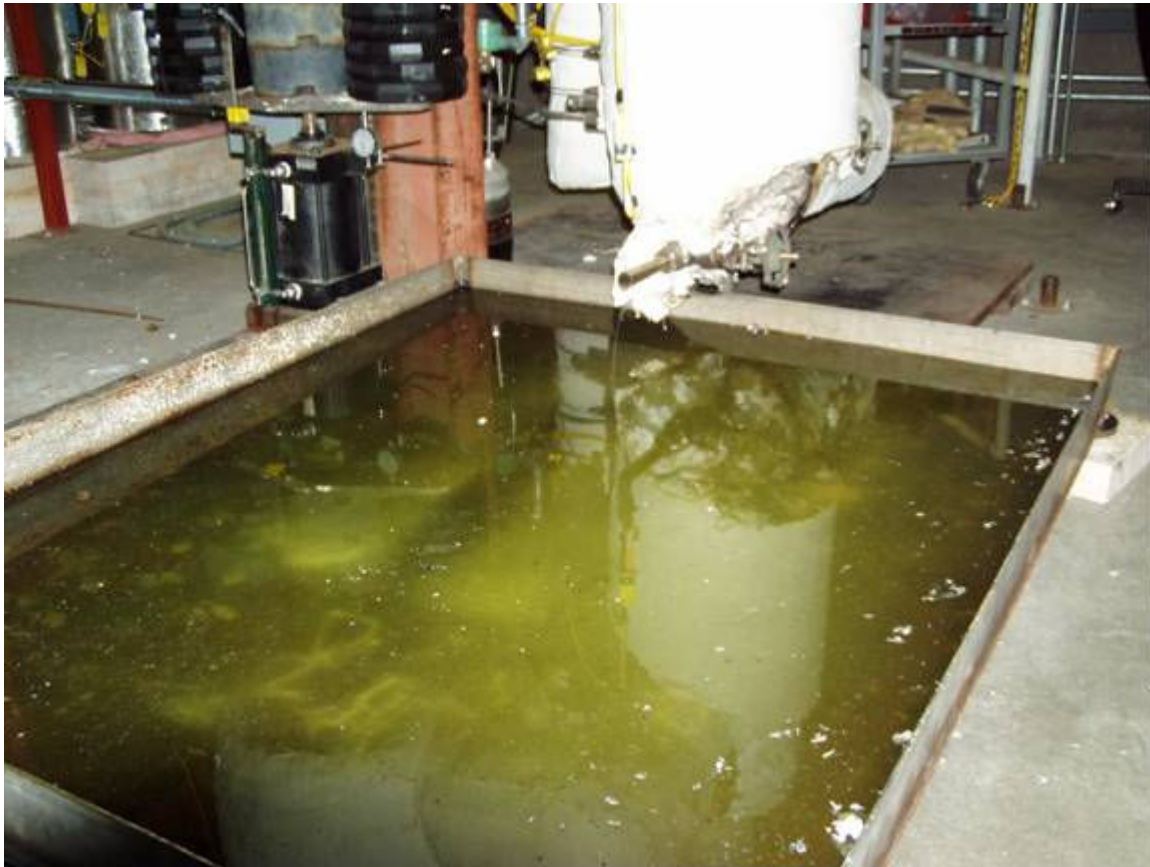
Figure 19 - Molten Salt Following System Draining
