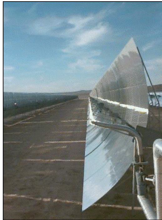
Figure 9. Row of LS-2 collectors at Kramer Junction
