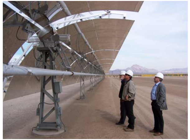
Figure 6, Nevada Solar 1 solar collector
