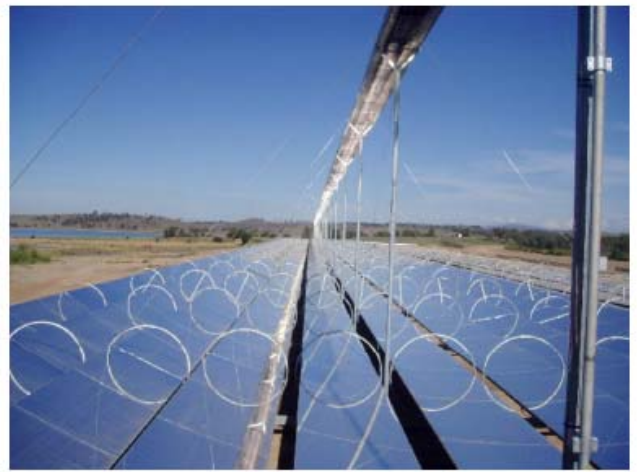
Figure 7: Linear Fresnel collector (Ausra)
