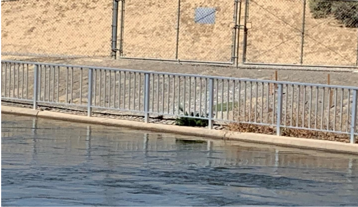
Figure 3-3. Section of the Aqueduct with reduced freeboard at high flows
