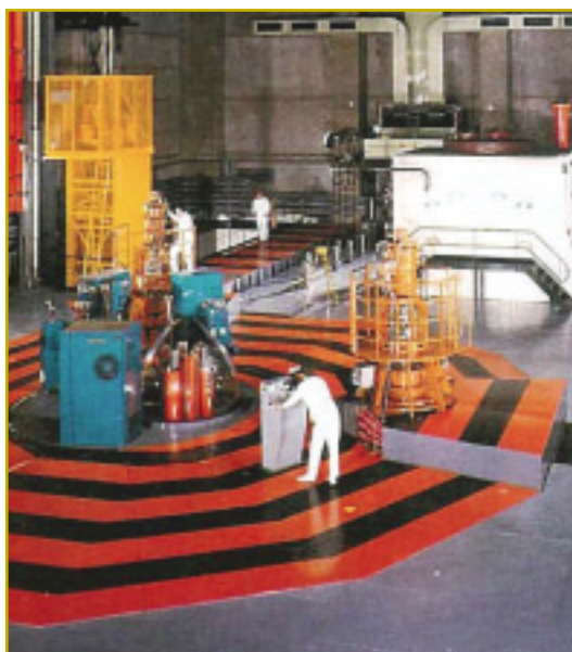
The hall of the reactor building
