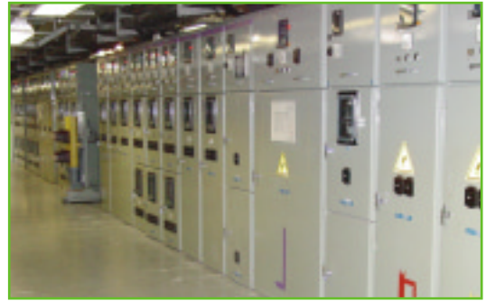
Electrical equipment cabinets
