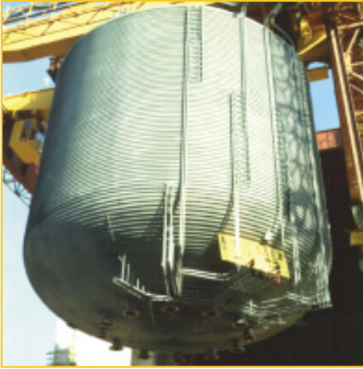
The primary containment enters the reactor building
