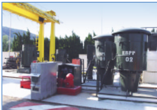
Pumping station, external view
