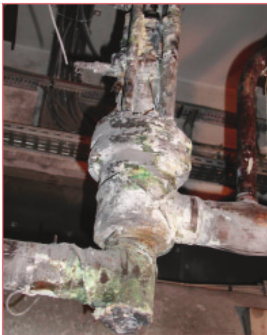
Valve with insulation removed after a sodium leak
