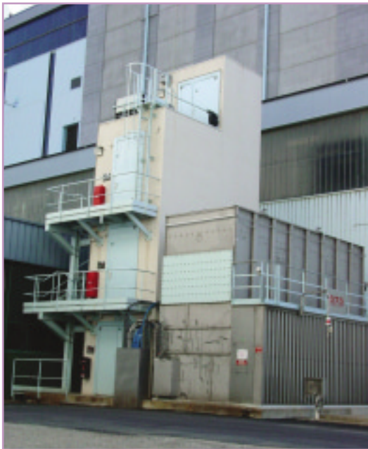
Emergency cooling system air cooler (on the right, near the pump room)
