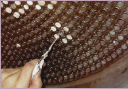
Inspecting the tubes of an intermediate heat exchanger
