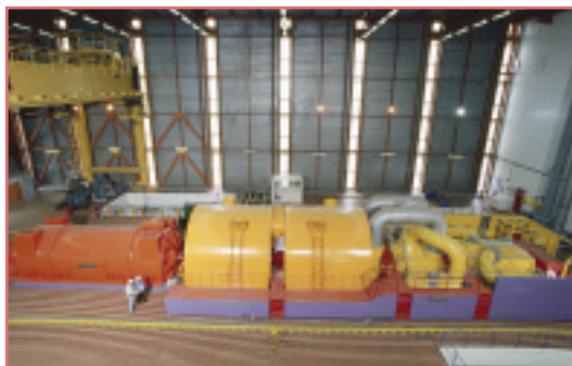
The turbo-generator set
