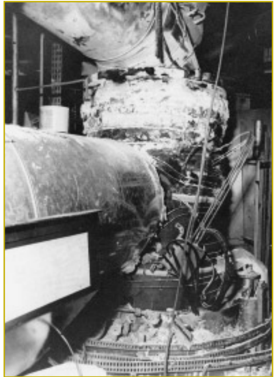
Heat exchanger with insulation removed after a sodium leak
