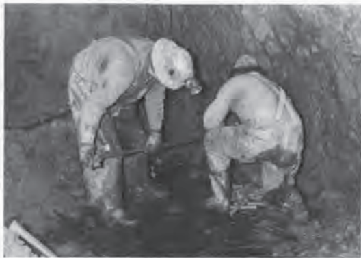
At the Rico mine in Colorado John Martinez (right) loads charge in the rock face while Willy Akeha, miner, waits to tamp it into place. Photograph by Ralph Leubben, 1953.
