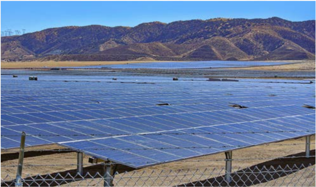
Solverde1 Solar Plant located in Lancaster, California.
