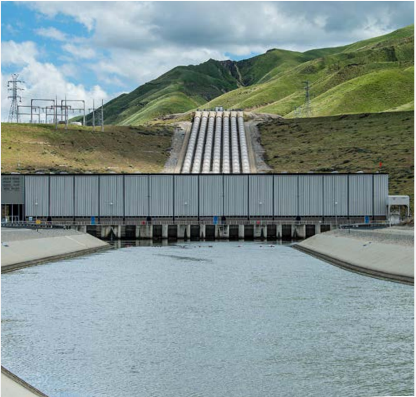
Teerink Pumping Plant, part of the California State Water Project, is located in Kern County.
