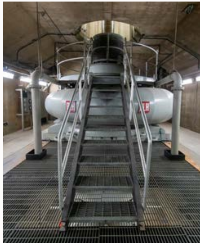
Edmonton Pumping Plants pumps elevate State Water Project water nearly 2,000 feet over the Tehachapi Mountains to Southern California.
