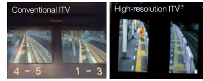
Installation of high-resolution ITVs
