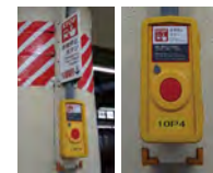
Emergency stop buttons on platforms
