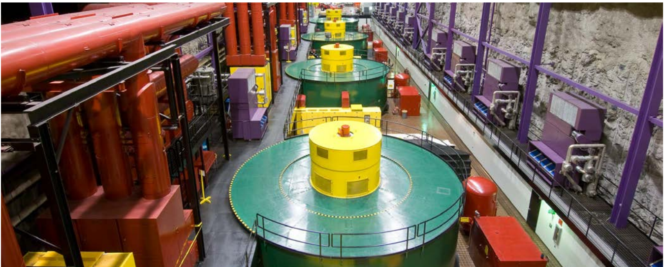
Figure 17-3 — Typical Hydroelectric Power Turbine Hall
