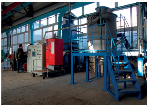
Figure 5. The reactor module body for plasma-steam-oxygen waste treatment in the stage of its installation.
