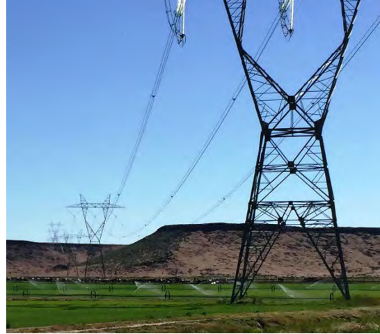
500-kilovolt (kV) transmission line near Melba, Idaho
