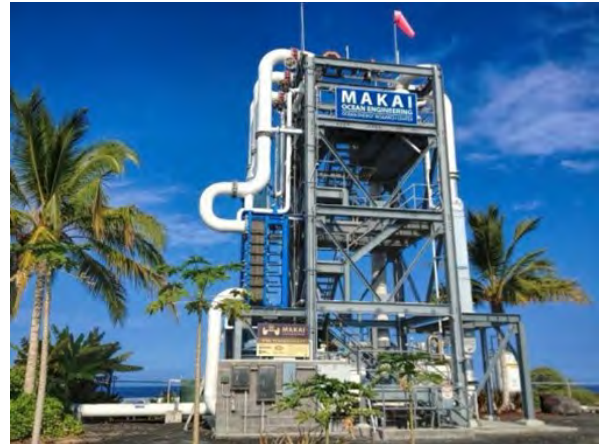
OTEC Pilot Project, Keahole Point, Kona
