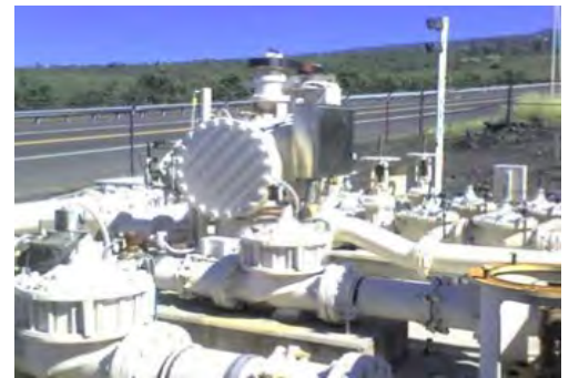
Hawaii County Dept. of Water Supply's 45 kW in-line hydro plant in Kona, Hawaii
