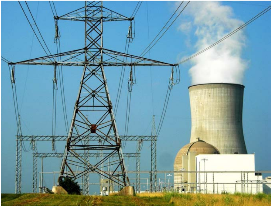
FIG. V-4. Power lines coming into the Callaway NPP.
