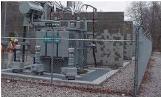
AUTO-TRANSFORMERS WITH FIRE WALLS
