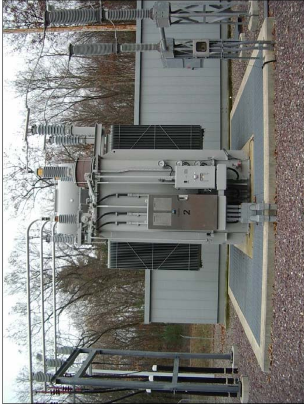
Figure 2.3-18 115-50kV (2x25kV) PRIMARY TRANSFORMER (40 MVA) CALTRAIN ELECTRIFICATION PROGRAM
