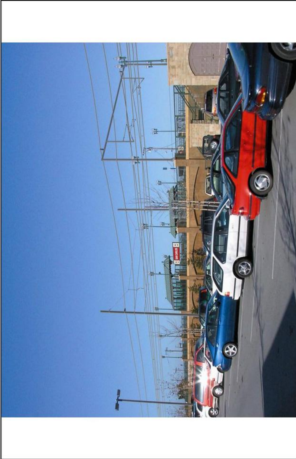
Figure 3.1-5 VIEW TO SAN CARLOS STATION PLATFORM WITH OCS SYSTEM, HEADSPAN AND PORTAL ARRANGEMENT CALTRAIN ELECTRIFICATION PROGRAM
