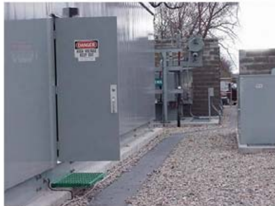
CONTROL BUILDING AND AUTO-TRANSFORMER
