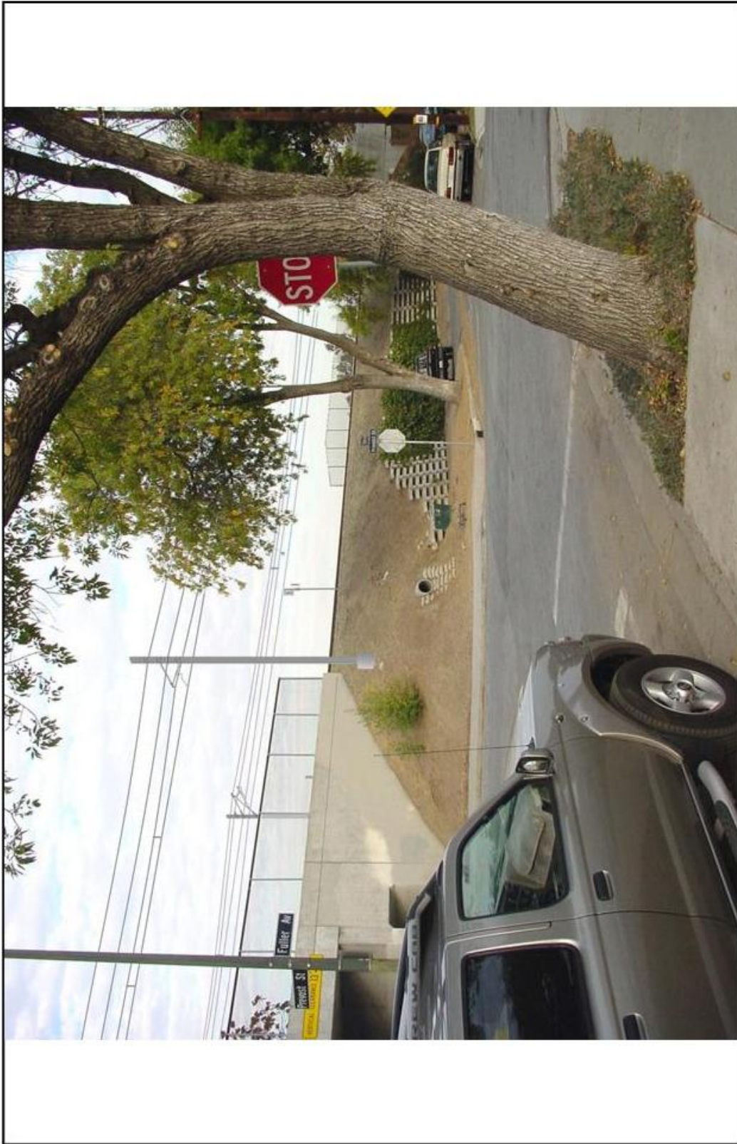
Figure 3.1-11 VIEW FROM SOUTH SAN JOSE RESIDENTIAL AREA TO ELEVATED RAILROAD CORRIDOR WITH OCS SYSTEM AND SIDE POLE CONSTRUCTION CALTRAIN ELECTRIFICATION PROGRAM
