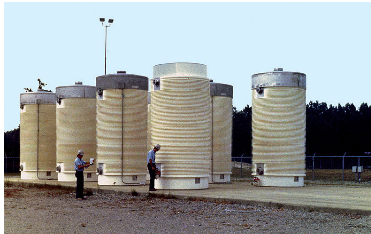
Dry Storage Facilities
