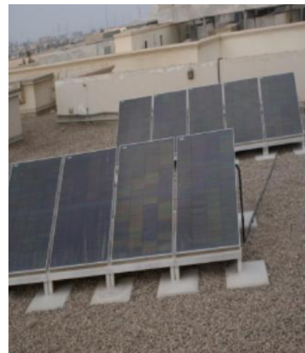
(a) (b) Figure 1: (a) A dusty day in the golf, (b) Roof-top panels affected by dust [12].
