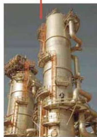
Separation at amine contactor towers
